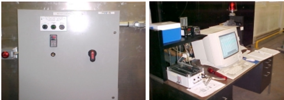
Figure 3. The Heater Control Panel
